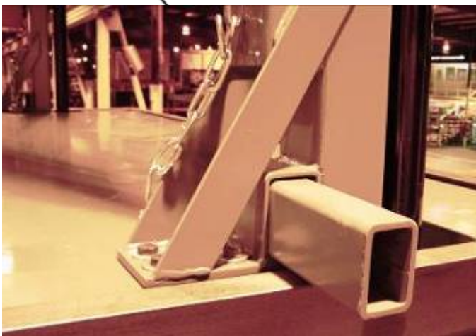
Figure 11 Maintenance Devices – Typical (4) Corners
